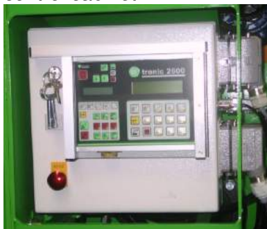
Emergency off button on the control cabinet
