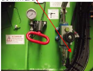
Switch valve level downwards
