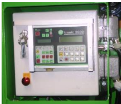
Emergency off button on the control cabinet
