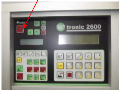
Emergency off key on the control cabinet
