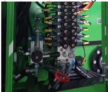
Switch valve level to right
