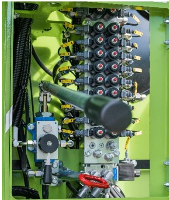
Switch valve level downwards
