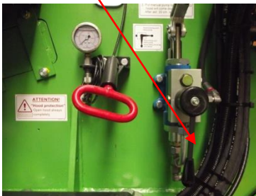
Switch valve level downwards
